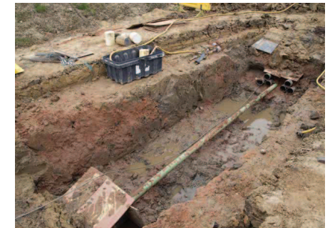
6. Excavate Joint Pit and Conduct Cable Pull (Post Duct Installation and Reinstatement)
